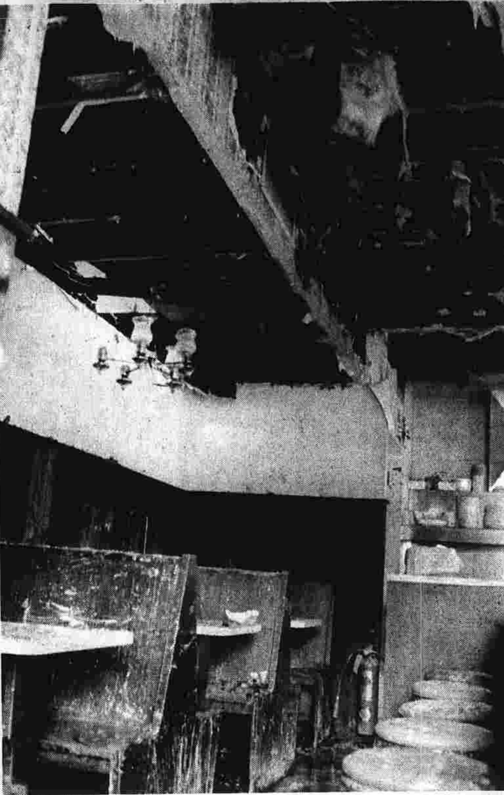
The interior of Childer's Restaurant at 250 Hartford Rd. was badly damaged this morning by a fire which apparently started in the furnace. The cause of the blaze is being investigated. (Herald photo by Oflara)
